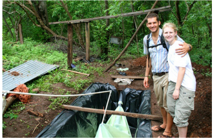
Director of Operations Wes Meier and Marketing Director Megan Sellheim after the completion of a biodigester installation in El Valle de San Antonio for the 20x20 project. May 2010.
