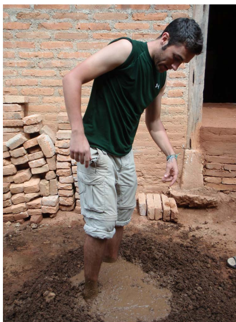
Here Greg is mixing up the mortar before the construction of a fuel-efficient oven in Nicaragua.
